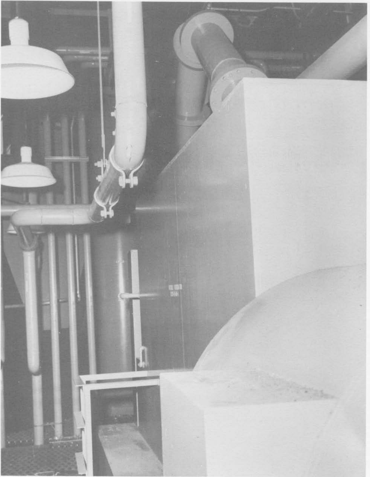
Piping on west side of diesel generator (Neg. No. 61633A dated 1-5-61).
