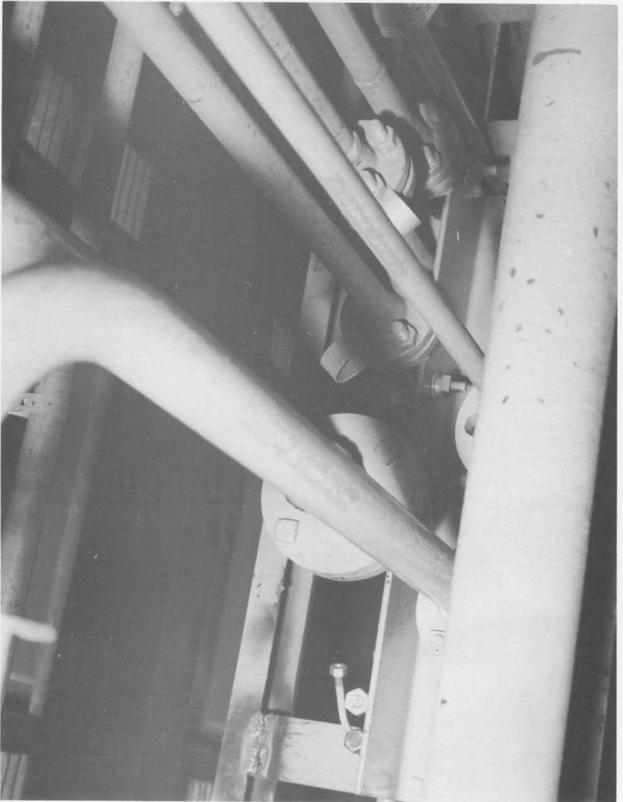
Pressurization control unit facility interface Quad 3 below Level 8 (Neg. No. 67367A dated 4-14-61).
