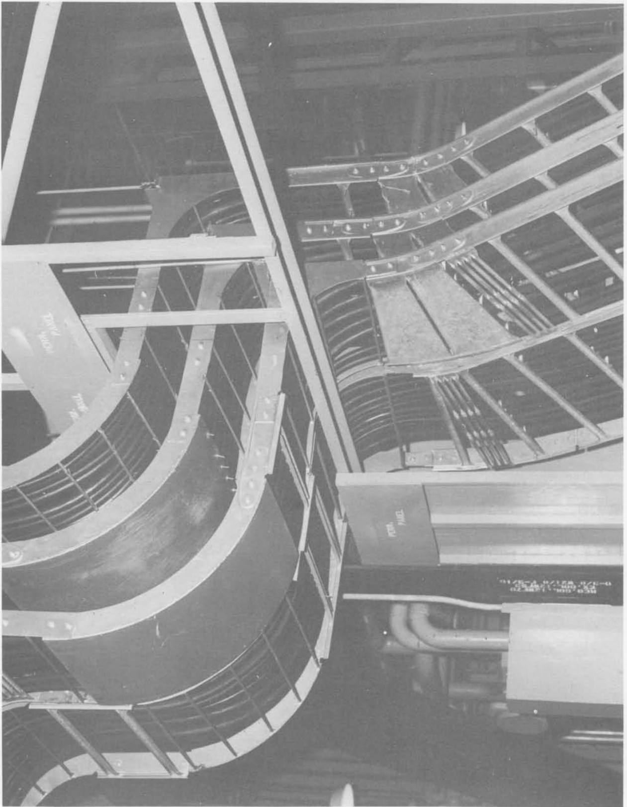
Umbilical loop shown extending through missile enclosure panels (Neg. No. 67564A dated 4-19-61).
