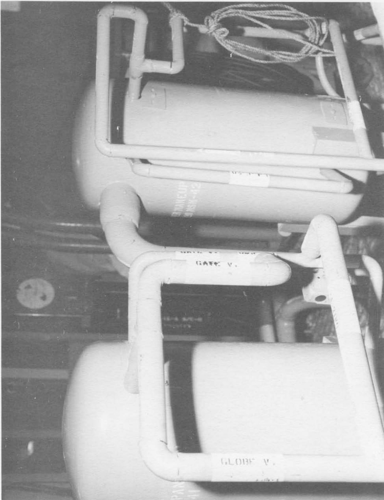
Chilled water and makeup tanks, Q-3, looking toward missile shaftway (Neg. No. 67554A dated 4-19-61).
