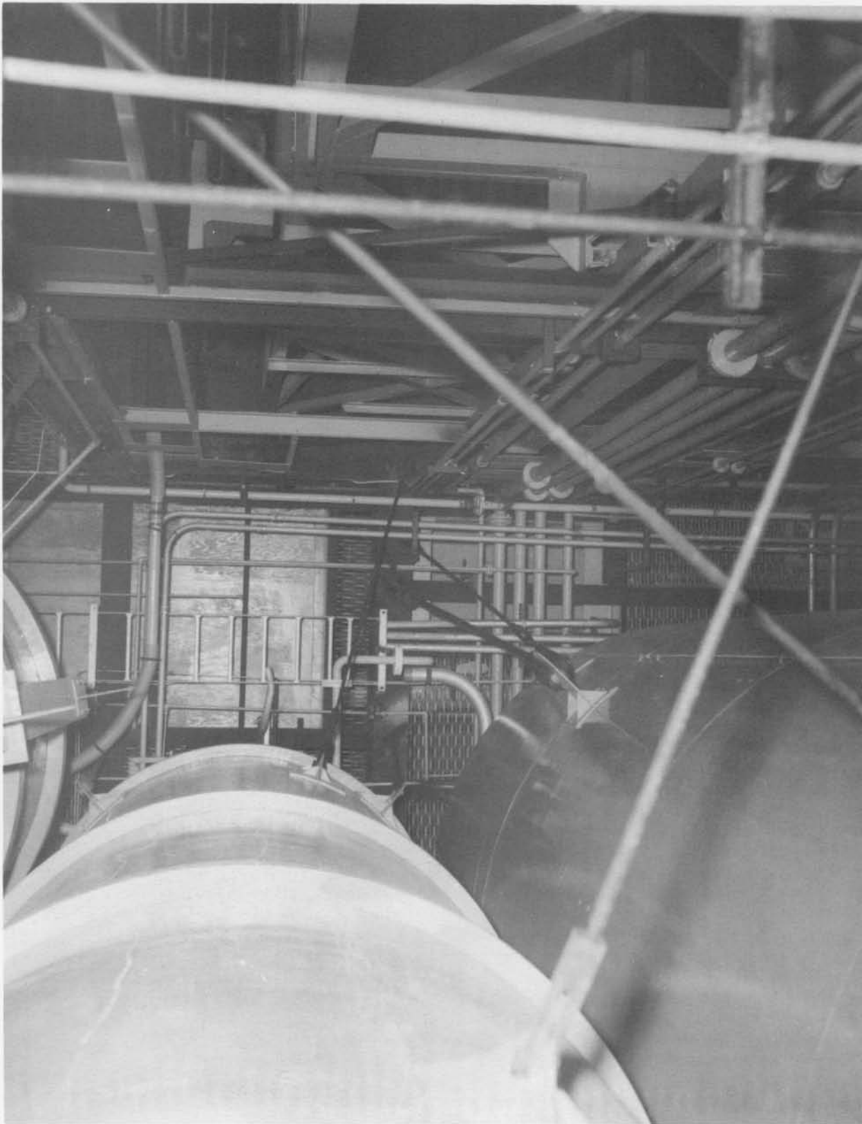
Looking up to Level 7 from near Column K (Neg. No. 68082A dated 4-27-61).
