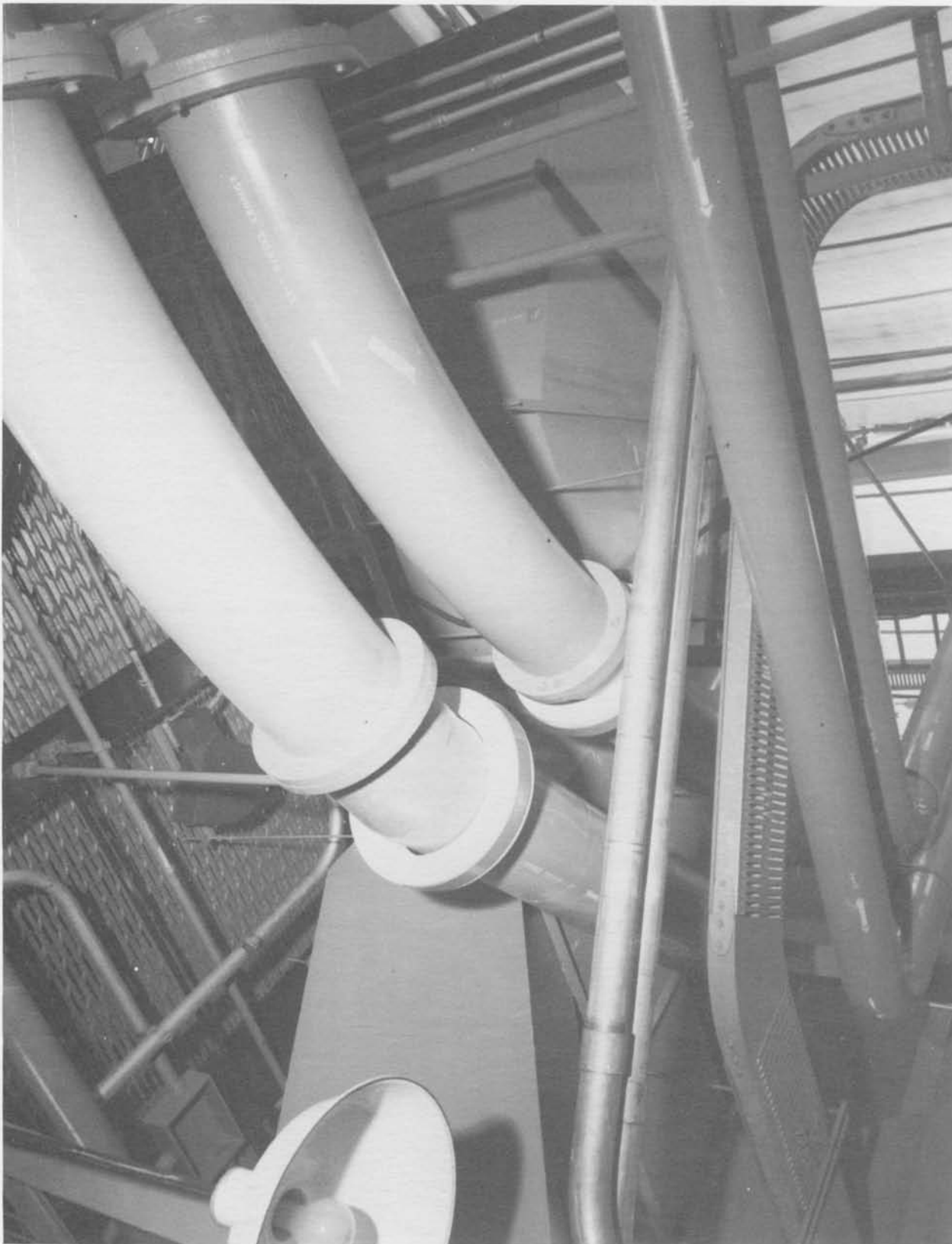
Twelve-inch diesel exhausts and ducting, looking up from elevator toward Column F (Neg. No. 68022A dated 4-26-61).
