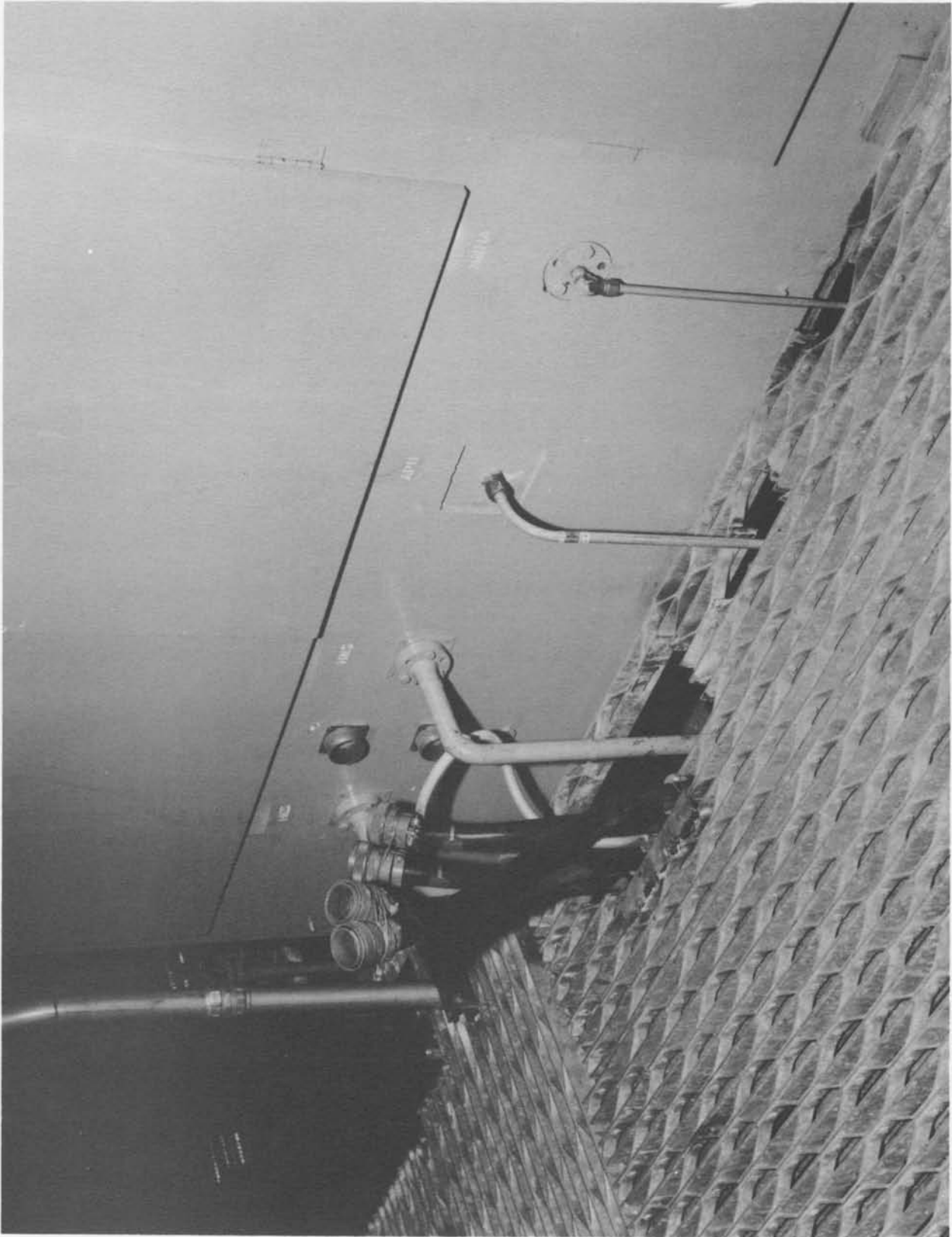
East side of interconnects of PDU (Neg. No. 67570A dated 4-19-61).
