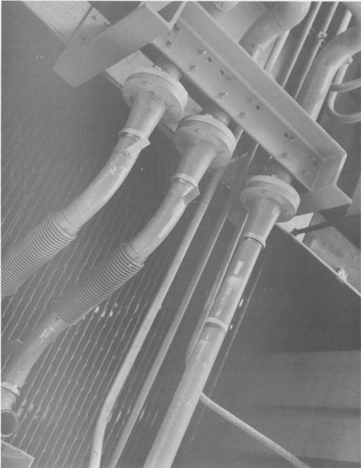
Power distribution unit facility interface Quad 3 below Level 8 (Neg. No. 67366A dated 4-14-61).
