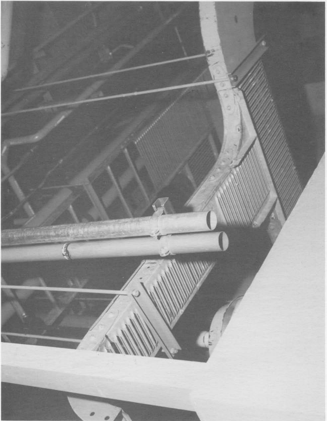
Showing proper routing of facility cable tray and conduit above nonessential and essential bus (Neg. No. 67561A dated 4-19-61).
