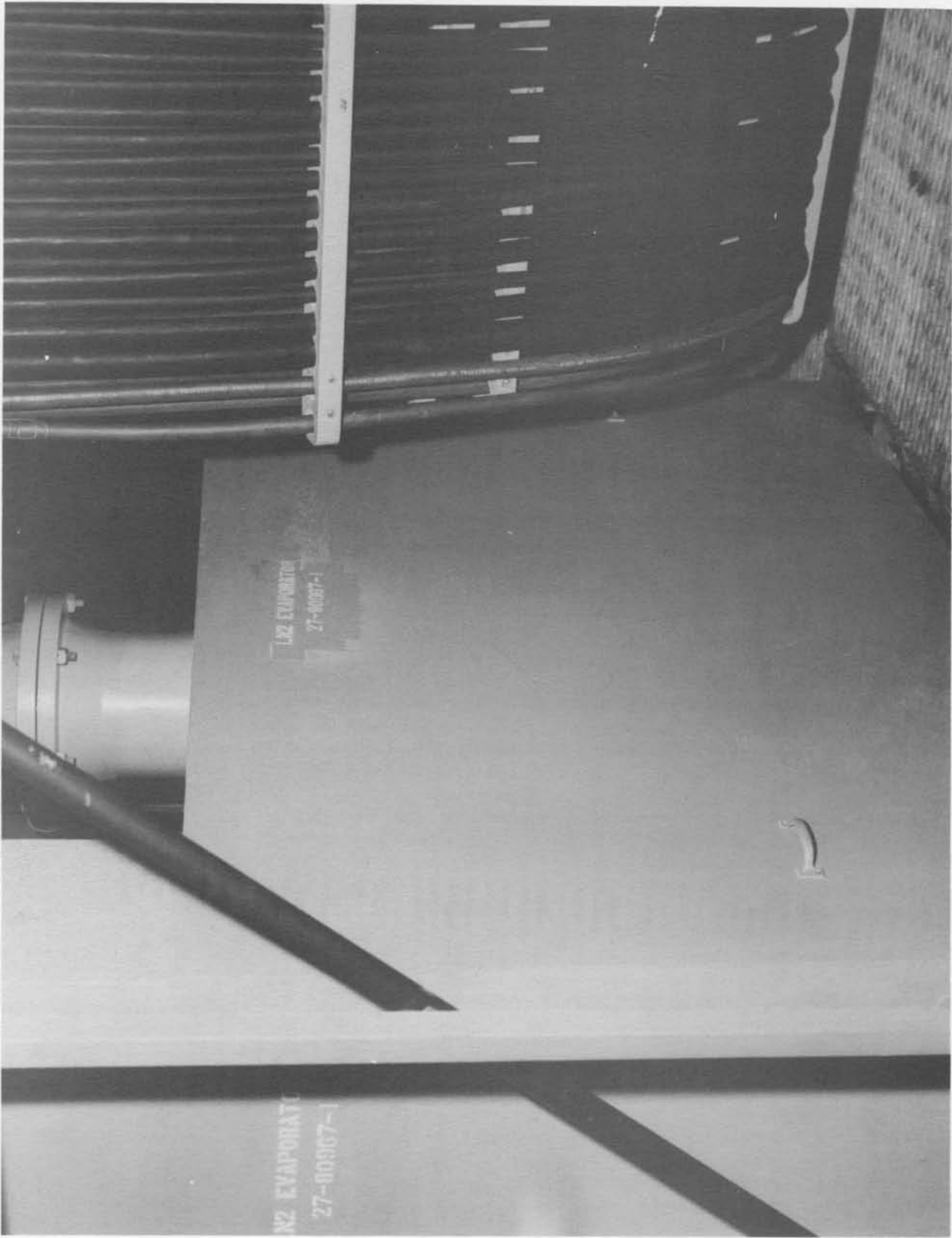
View of Quad 3 side of LN 2 evaporator tank (Neg. No. 67568A dated 4-19-61).
