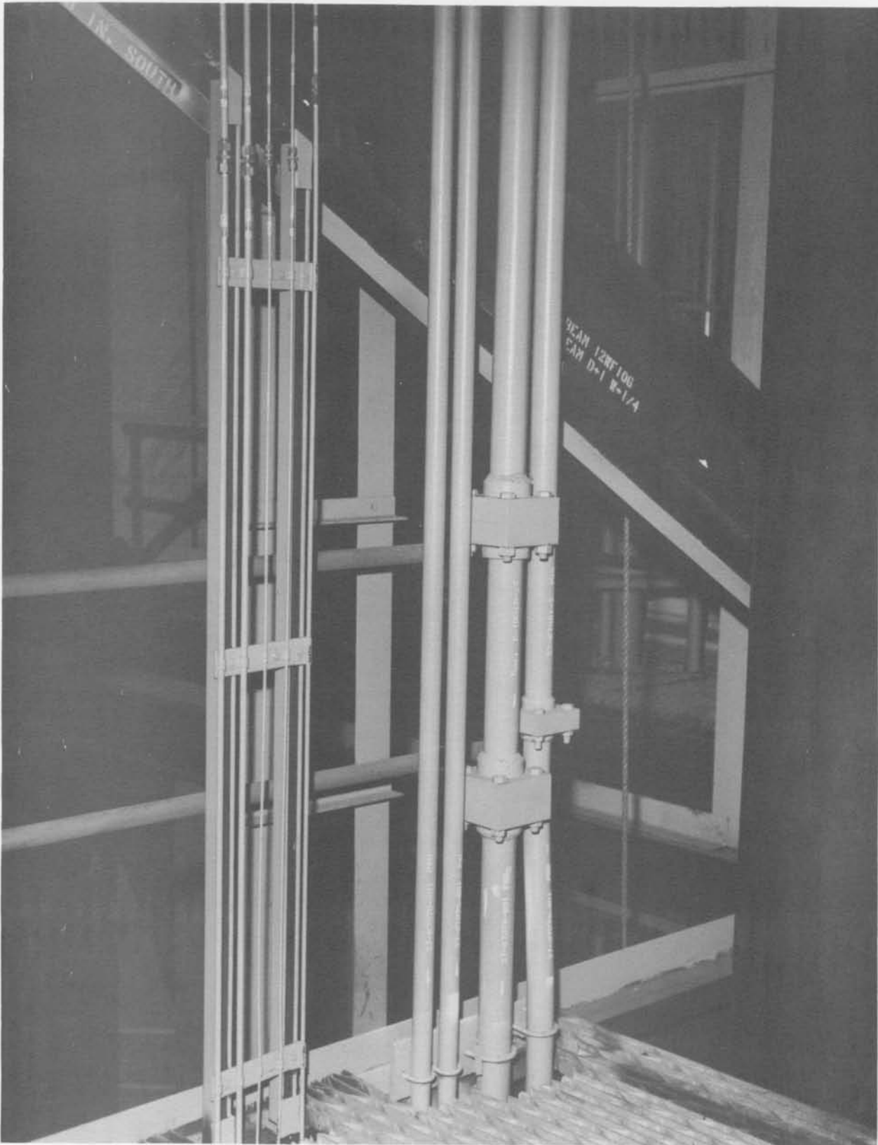
Vertical run, showing hydraulic pipes running through Level 4 (Neg. No. 67563A dated 4-19-61).
