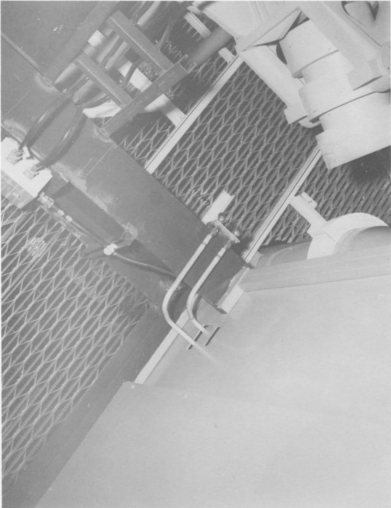
Hydraulic tubes to crib lock at Column D (Neg. No. 64932A dated 2-27-61).
