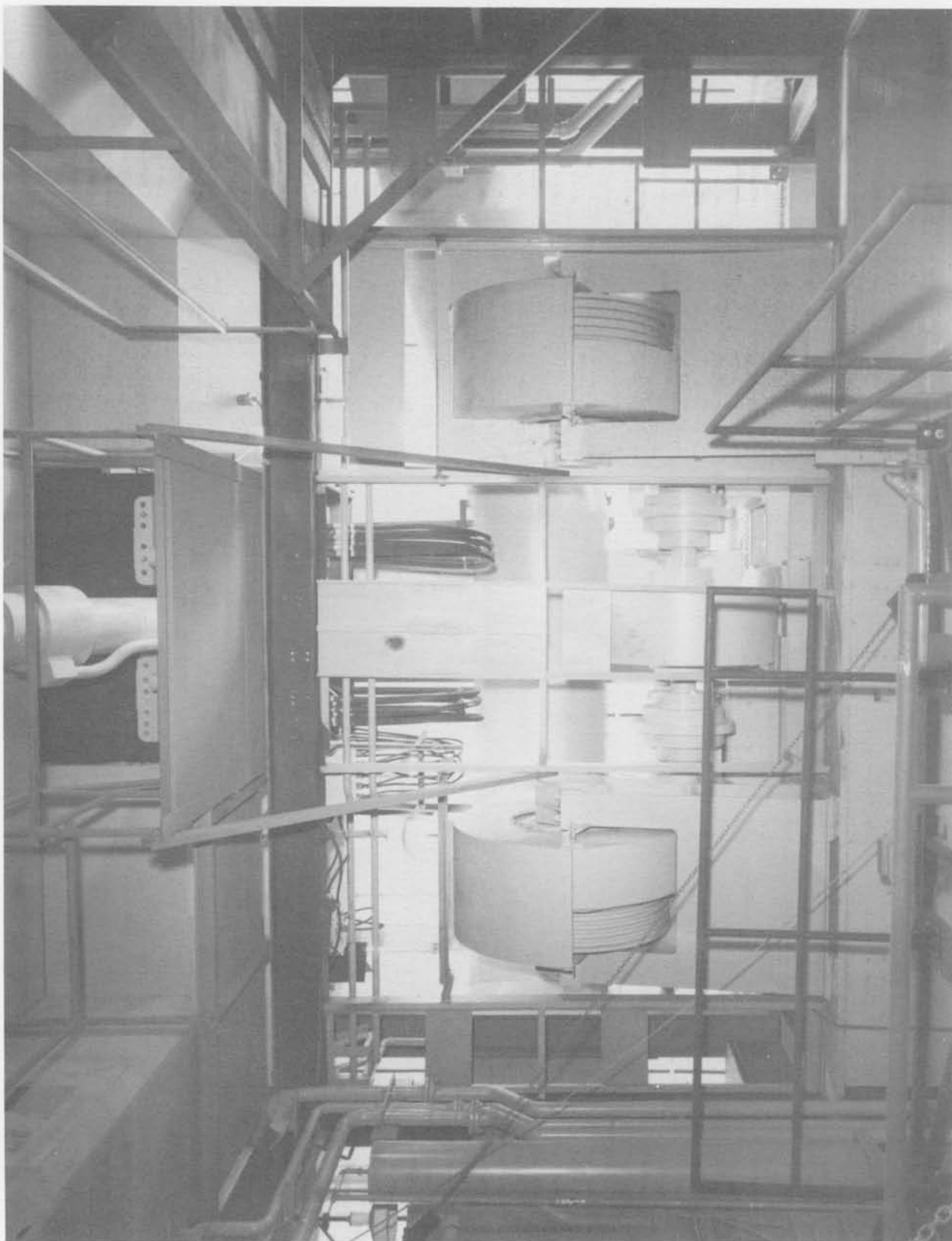
Drive mechanism at Column J to K, looking east (Neg. No. 68016A dated 4-26-61).
