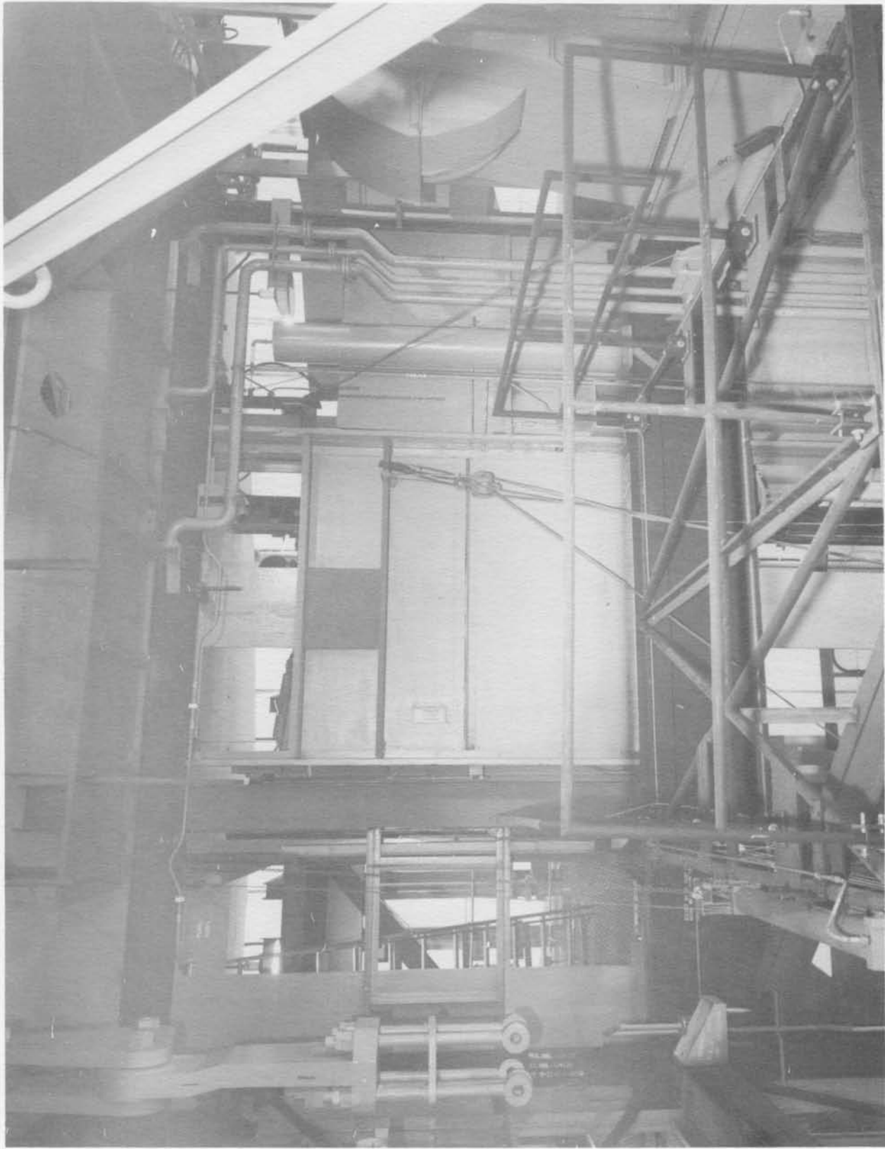
View of work safety platform at Column K to B-1, looking north (Neg. No. 68015A dated 4-26-61).
