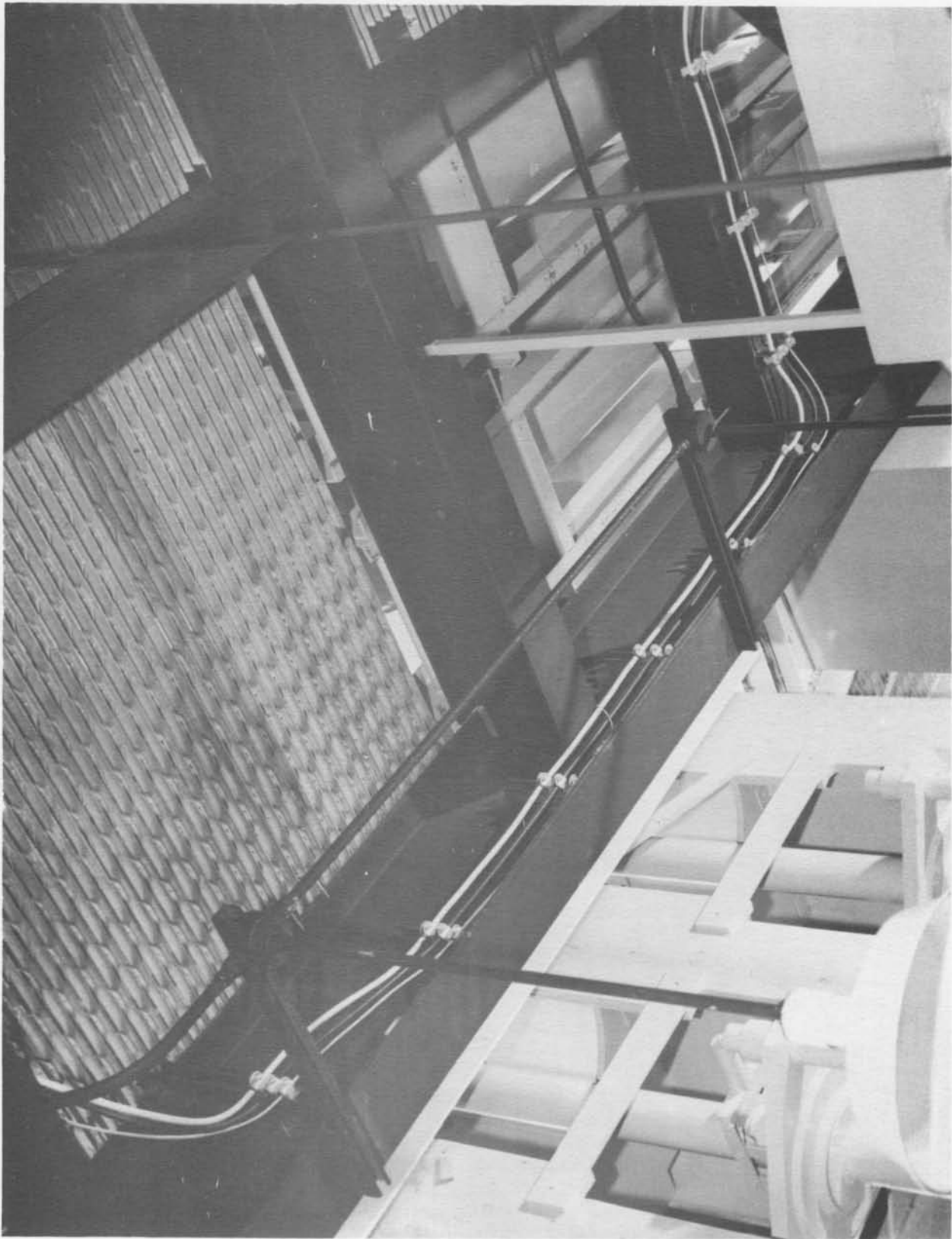
Cables to hydraulic reservoir (Neg. No. 56444A dated 10-7-60).
