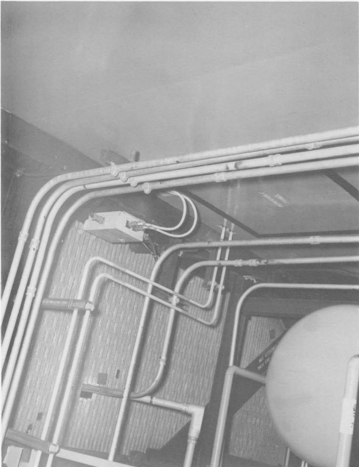
Hydraulic tubes to west crib lock (Neg. No. 64930A dated 2-27-61).
