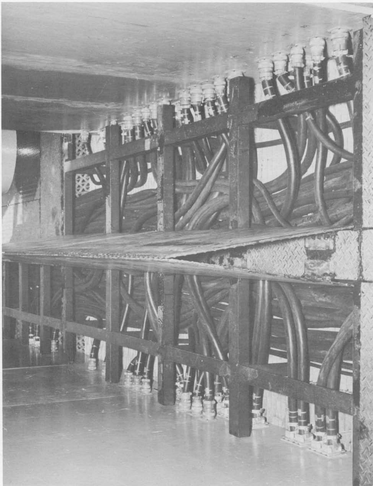
Cables under steel deck logic No. 1 to responder No. 1 (Neg. No. 55772A dated 9-27-60).
