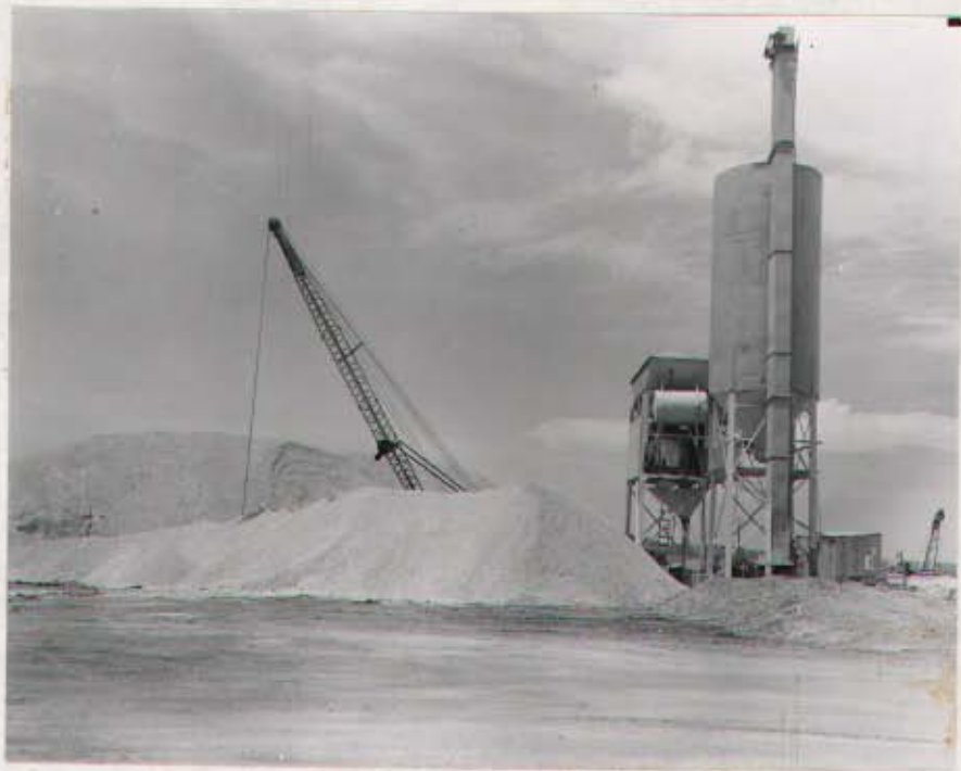
SITE 4. CORTLAND, NEBRASKA. 3 Aug. 60. View facing west shows general area of batch mixing plant. #39124.
