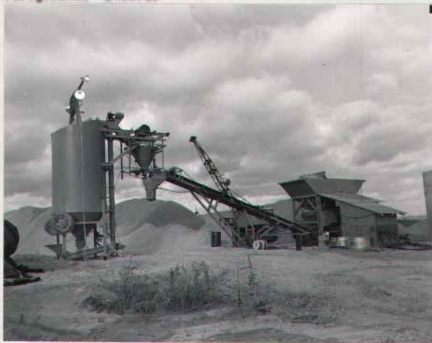
SITE 6. WILBER, NEBRASKA. 2 Nov 61. Northeast view shows closeup of batch plant. #41527.
