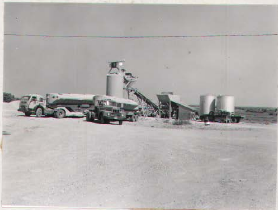
SITE 6. WILBER, NEBRASKA. 6 Oct 60. Northeast view shows Western Contracting Corporation batch plant at job site. Special trucks used for hauling cement in foreground. #40873.
