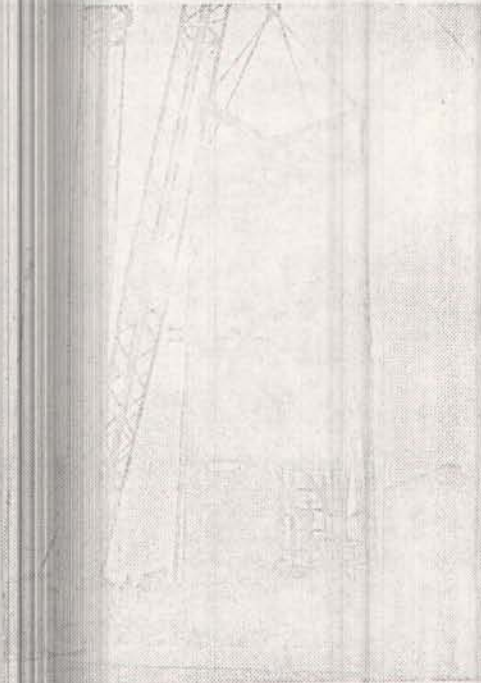
Platform in place at top of silo . . . Workmen lower structure inch by inch.
